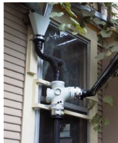
Programmable valve to divert a rain's first flow away from the cistern.
