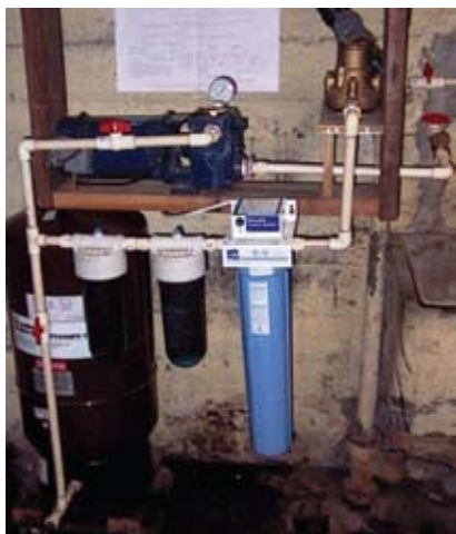
Purifying Rain water - Two particulate filters in series, rated at 20 and 5 micron particle size & an ultraviolet light sterilizer.
