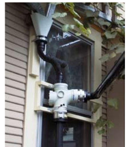
Programmable valve to divert a rain's first flow away from the cistern.
