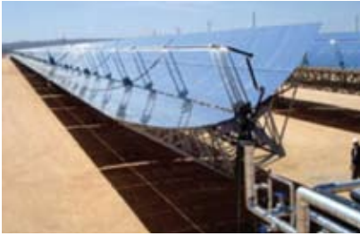
Parabolic mirrors concentrate heat to produce steam to run power turbines
